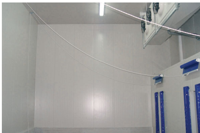
Refrigerated cells constructed with Isofrigo panels.
